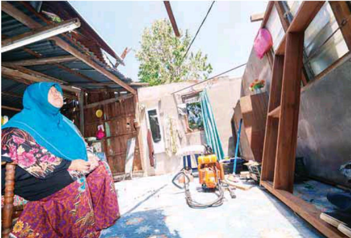
BLOWN AWAY ... Norfaezah Che Mansur looking at the sky from her living room after the roof of her house was ripped off during a storm in Kampung Permatang Sungkai in Kelantan yesterday. - BERNAMAPIC
