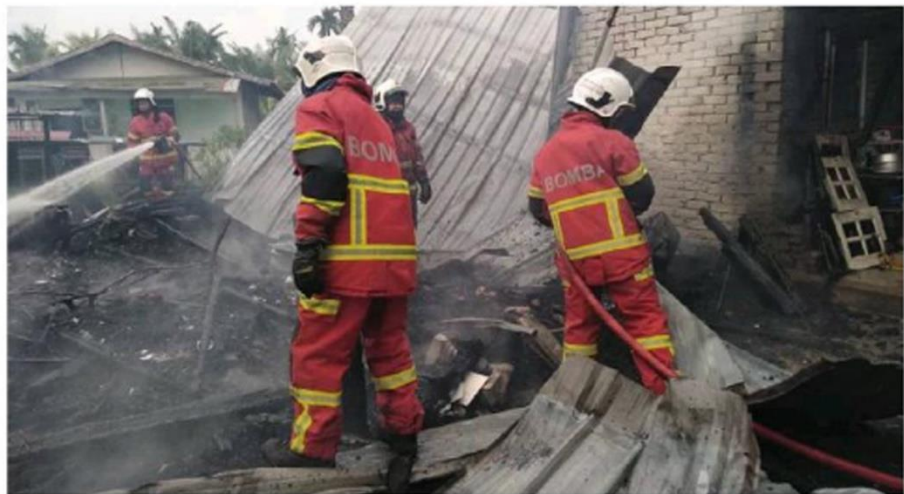
Firefighters conduct overhaul works at the razed house.
