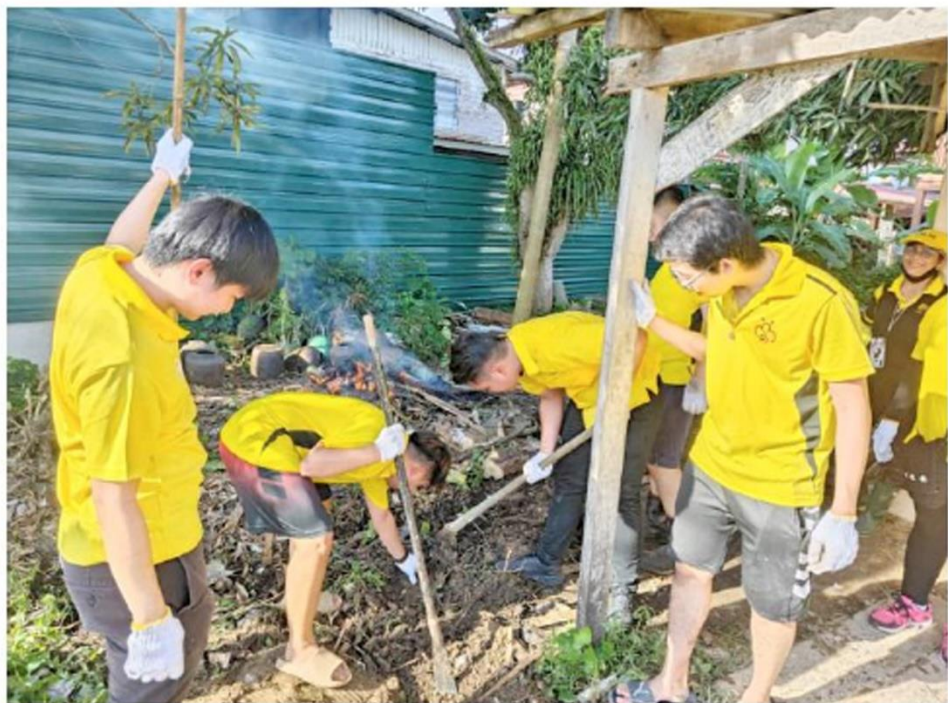
Pujut SUPP Youth members dig a drain around the house to allow better flow of water during heavy rain.
