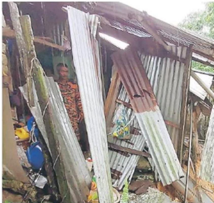
A firefighter inspects the landslide-damaged section of Rumah Imban.
