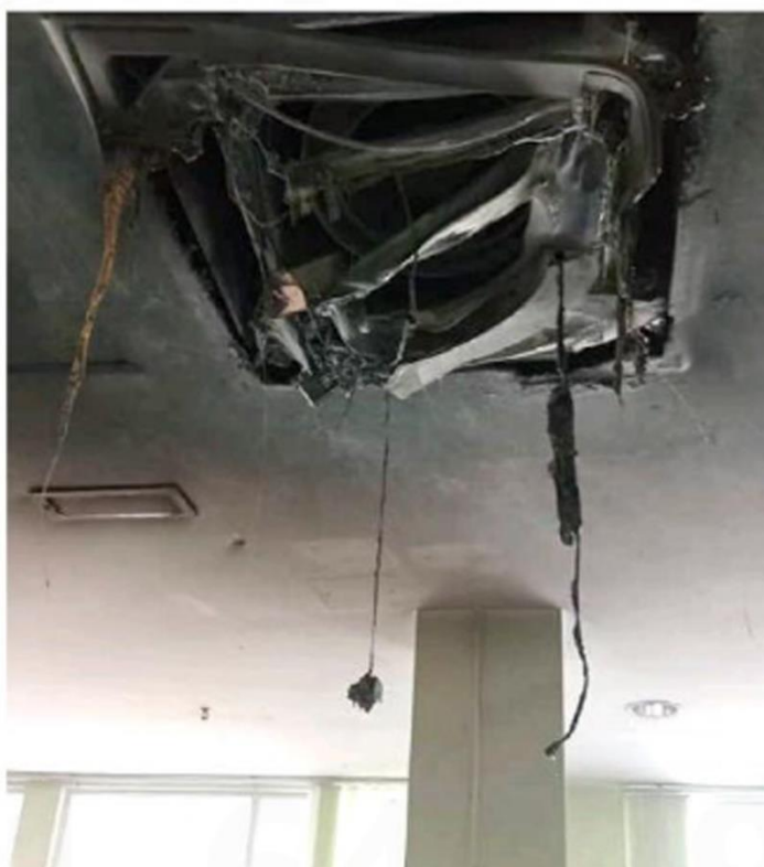
Handout photo shows the damaged air-conditioning unit.
